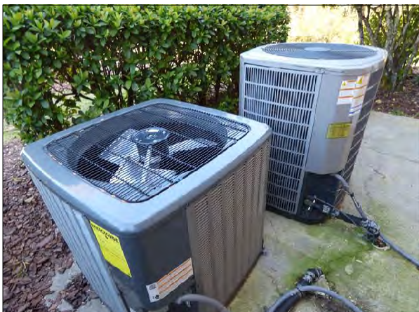
Nature Center HVAC
