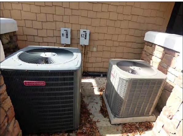
Activity Center HVAC
