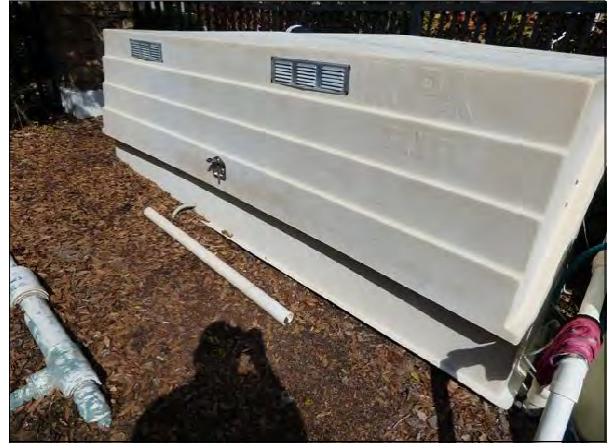
Pool Equipment Housing Boxes
